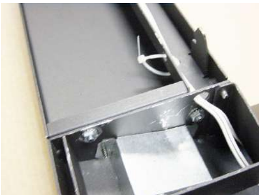
Figure 7: Wires secured with lock-tie
